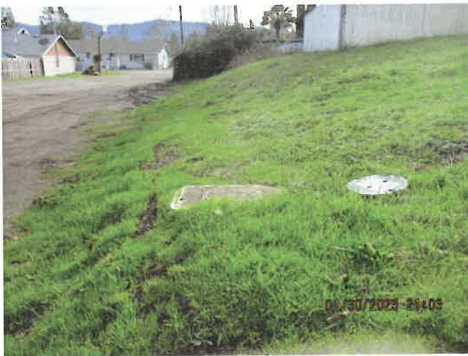
1780 NW Merle water meter (1)
