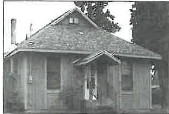
Incompatible vertical siding (T-1-11) has been placed over the original horizontal wood siding, changing the character of the house. This type of new siding treatment is not recommended.
