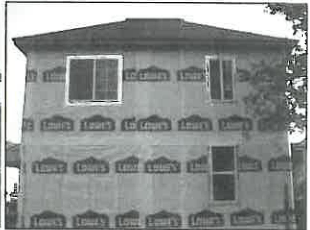
Incompatible replacement windows-not same size or type
