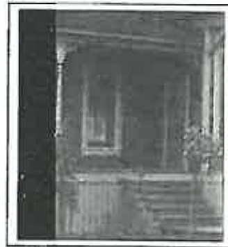
Vertical board skirting & jigsaw brackets on posts (Douglas County Museum No. GP.7240)
