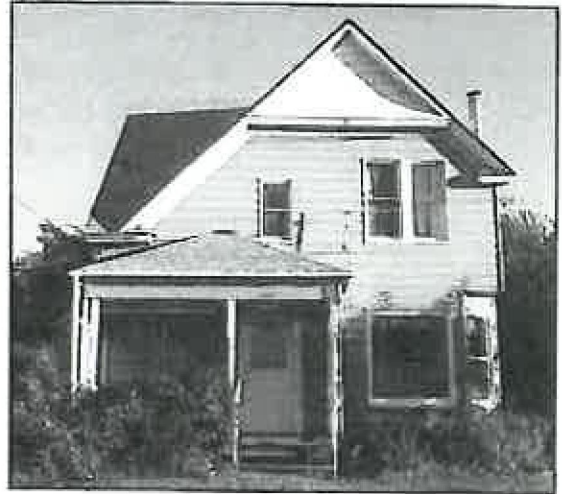
Wide metal siding replaced original narrower horizontal wood siding and original door and window trim were removed in 1970s. The loss of historic material and integrity is evident
