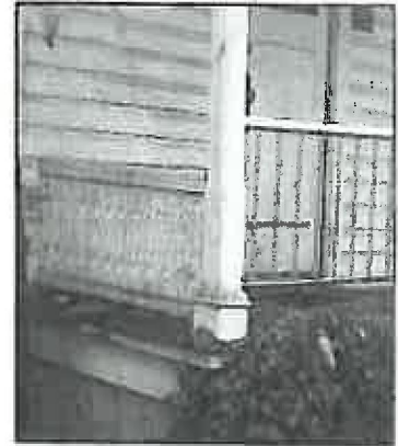
The original decorative railing on the left is lower in height and has closely spaced balusters. The incompatible replacement railing on the right is too high, has a top rail that is too "thin," and balusters spaced too far apart
