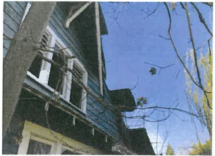
Eaves and roof caving in
