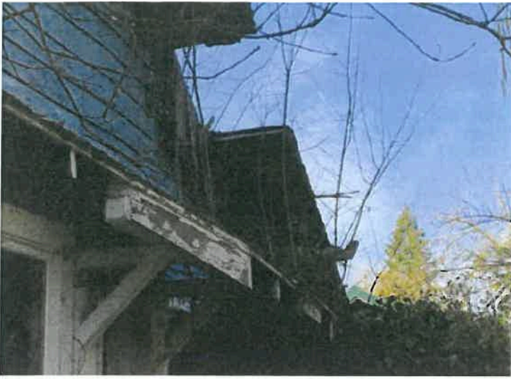
Fallen tree through rear house
