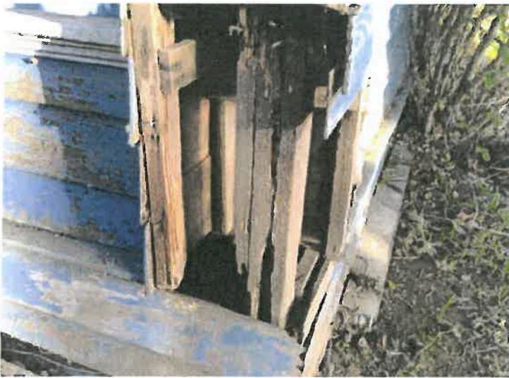
Rotting siding and foundation
