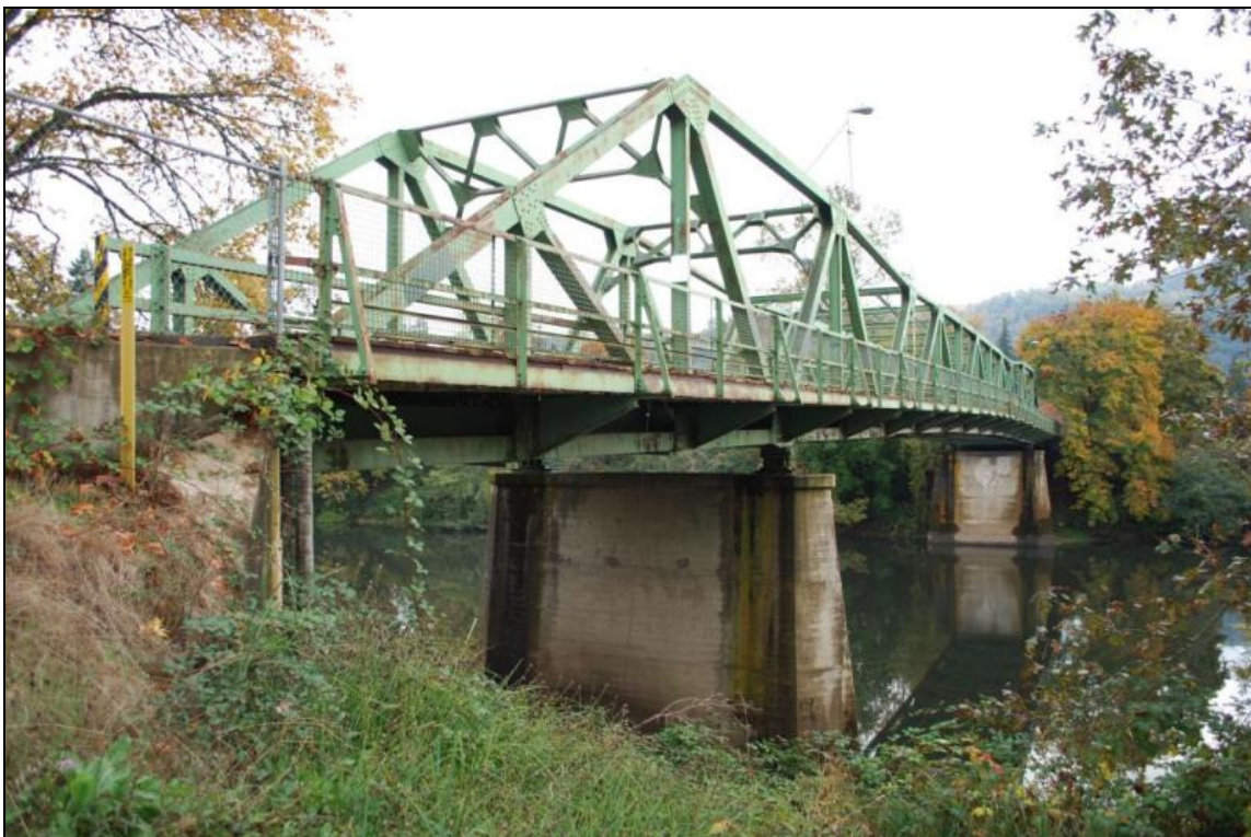
Photo 14 of 16: View to the southeast of the southwest elevation of the bridge (Resource G) over the South Umpqua River.
